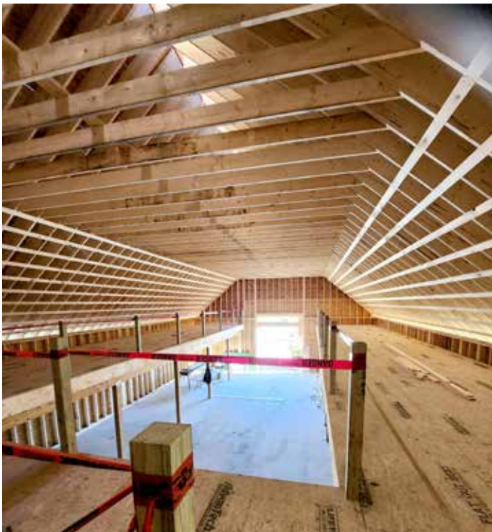
Sunlight permeates the interior of the West Gardiner Historical Society’s unfinished new building recently.
