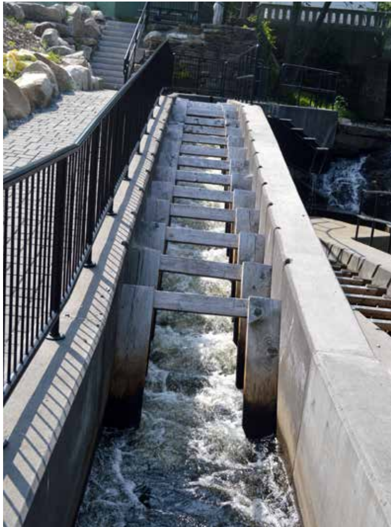
Water from Outlet Stream rushes through the fish ladder at the Box Mill Dam in North Vassalboro.
