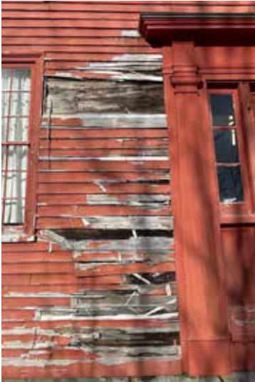
Gaps and cracks abound among the clapboards on the west side of the Maj. Reuben Colburn House in Pittston.
