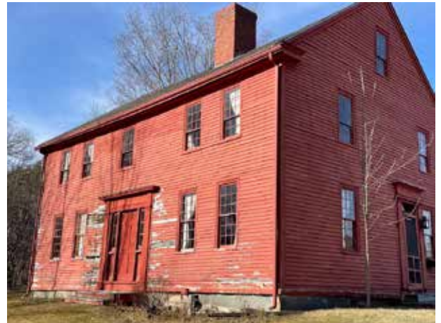
The Maj. Reuben Colburn House, on a state historic site located in Pittston, shows evidence of storm damage in this photo taken in early March of the building's west side, which faces the Kennebec River.
