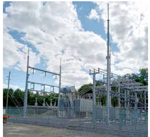
This electrical equipment standing on Route 139 in Unity Township is part of the Three Corners Solar Project.
